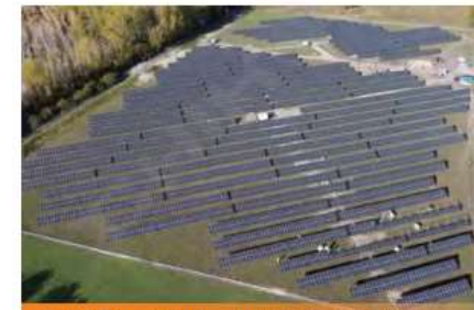
Project Size: 12MW Installation Site: Hungary
