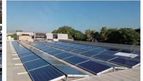
Project Size: 650KW Installation Site: UAE
