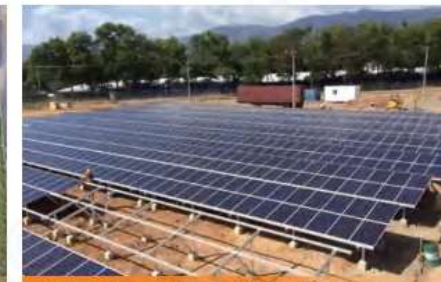
Project Size: 1MW Installation Site: Panama
